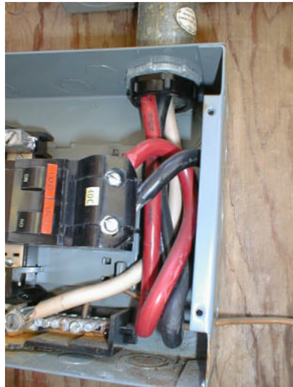
Figure 1 – Insufficient wire bending space
